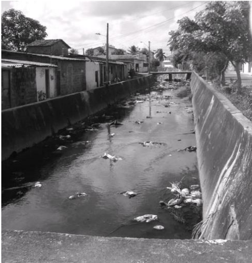
[Figure 1. Open sewer located in Pan-Americano neighborhood.]
